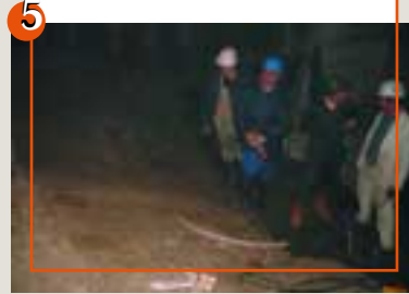
Picture 5: A slip plane observed during the excavation of the starting chambers
